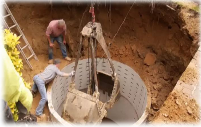
An OSHA-provided photo of a septic liner installation just before a fatal excavation collapse.
